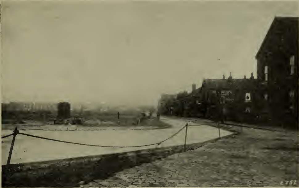
BEZA STREET, LEEDS, SHOWING HALF WIDTH CONSTRUCTION AND PROJECTING REINFORCEMENT AT JOINT.
